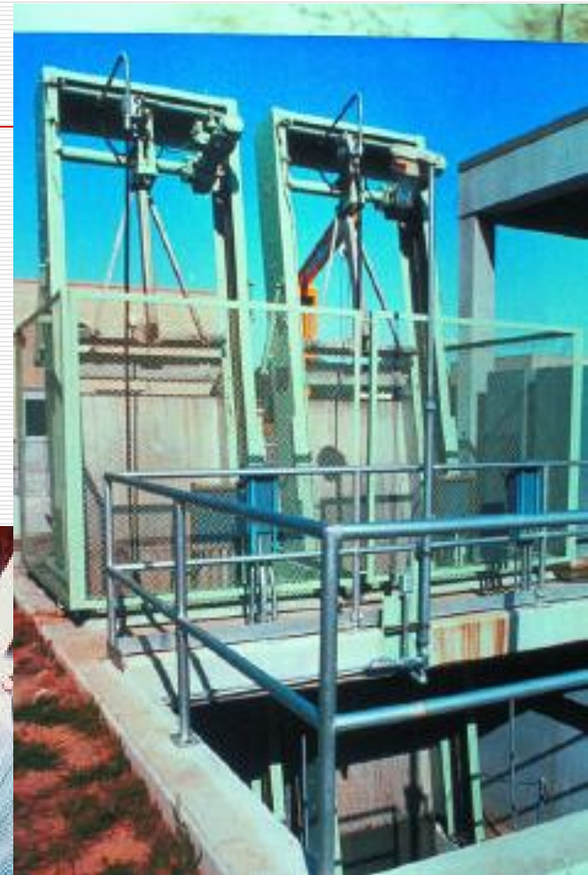
Figure 270. Vertical grab bar screens.
